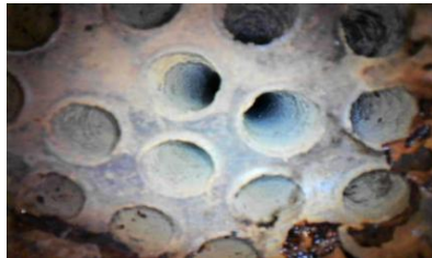
Fig 2a: Before DCI Treatment-tube side
