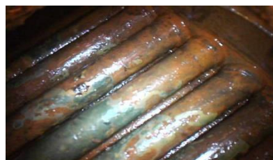
Fig 3a: Before DCI Treatment-shell side
